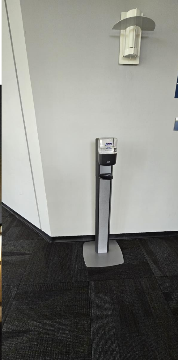
Automatic Hand Sanitizing Stations.
